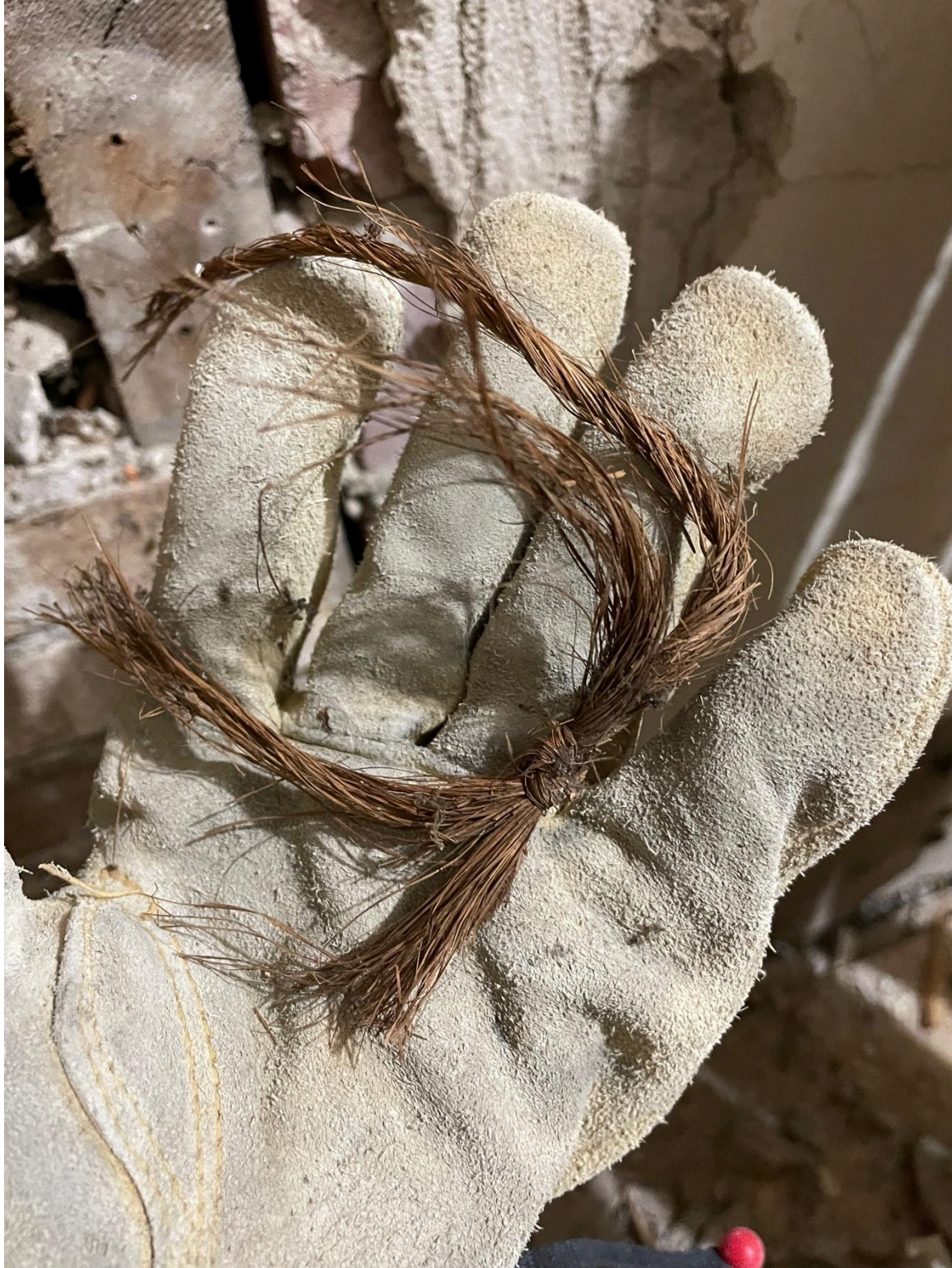
Figure 24 Artifact Braided Horse Hair Found in Failing Plaster Walls. Horse Hair Originally Used to Strengthen the Plaster Creating a Fibrous Network for the Material to Adhere to. Modern Methods Include the Addition of Fiberglass or Similar Material.
